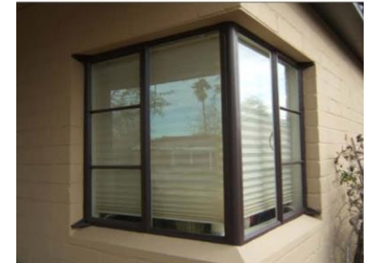
Low-e glass replacement (before and after). Courtesy City of Phoenix, Planning and Development Department, Historic Preservation Office.
